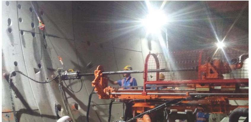
Sigra managed pressure drilling equipment installed for cross tunnel drilling and consolidation grouting. Lantang Tunnel, Hong Kong
