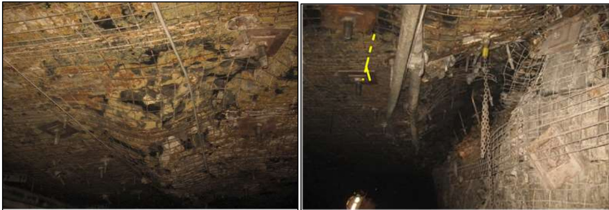
Figure 8. Austar gateroad centreline bagging and chain pillar side guttering near bent tendons (Moodie, 2011)
