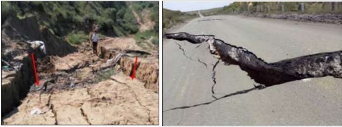
Figure 15. Bulianta LW22307 surface subsidence and cracking (Yang, 2019)
