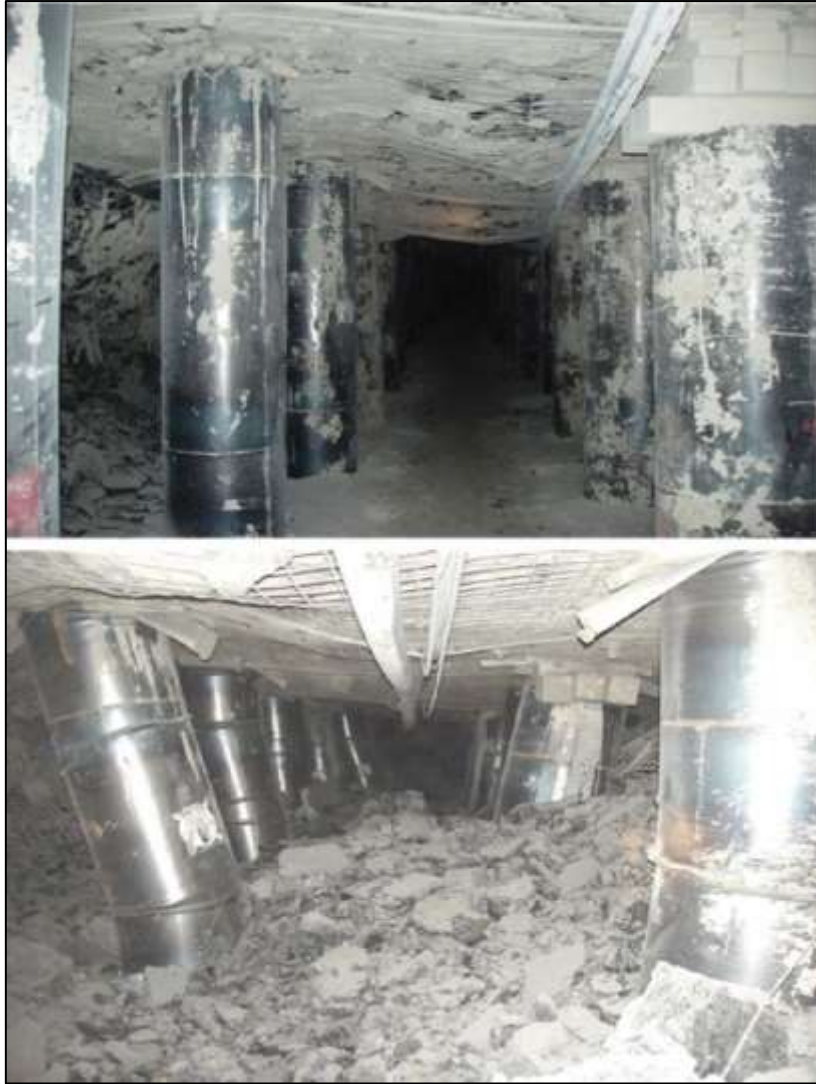
Figure 2: Effect of a coal burst on a gateroad before (top) and after (below) (Mark from an unspecified US mine in the North Fork Valley, 2016)
