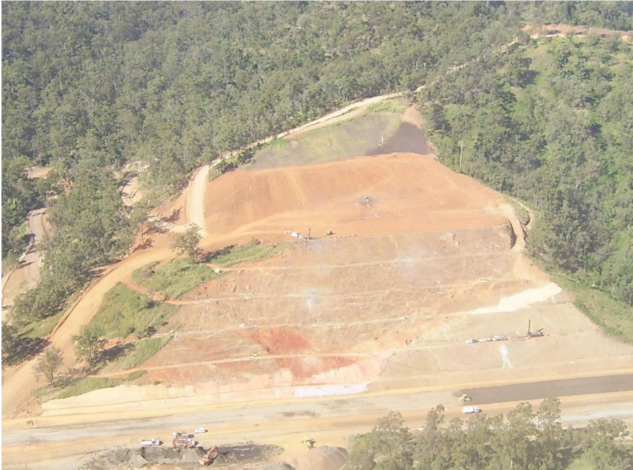
Figure 2 Aerial photograph of cut 3 during removal of the top of the slope and filling of the toe
